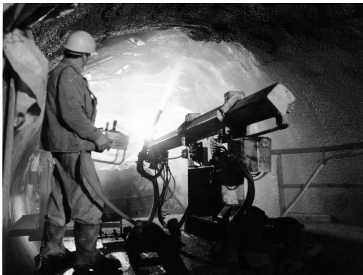
Figure 42: Tailor-made solution by MBT: The MEYCO® Robojet spraying manipulator is integrated into a small diameter TBM.
