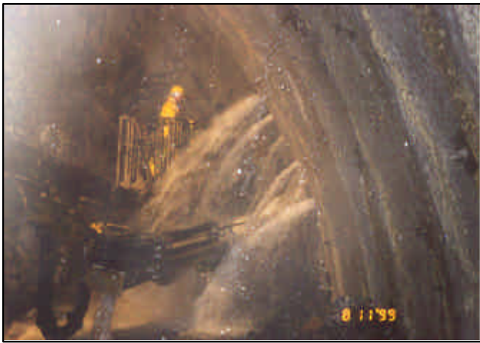
Figure 11: Meyco SA-170 alkali-free accelerated sprayed concrete to control active ground water, Blisadonna Tunnel, Austria, 2000
